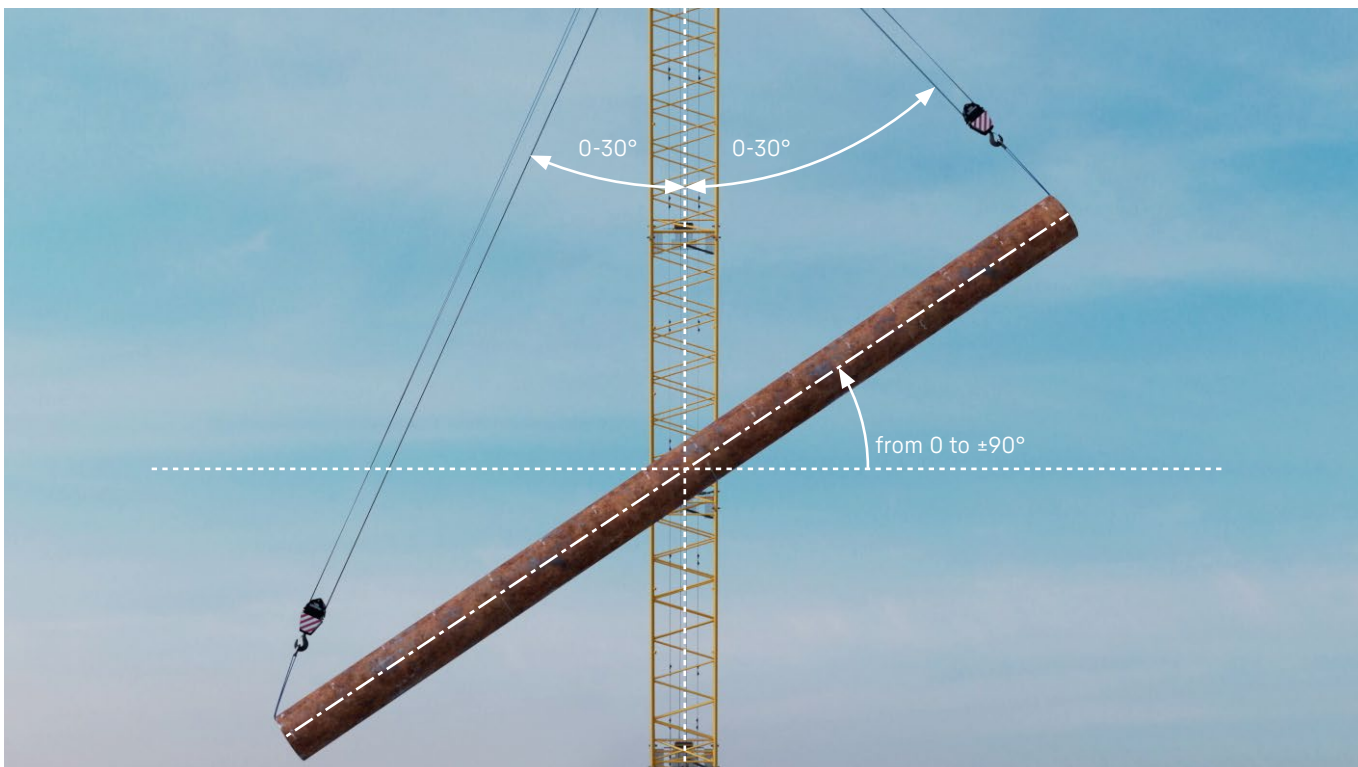
The pile can be continuously rotated into any position and held there, pile weight max. 90 tonnes.
