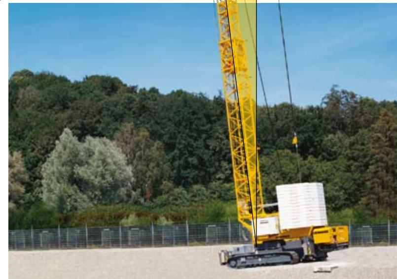
... and longitudinal inclinations up to 10% - no problem at all for Liebherr crawler cranes.
