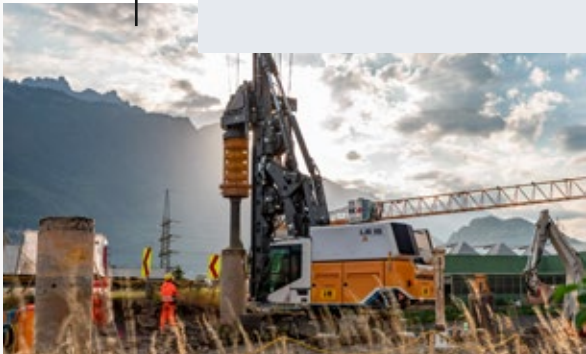
All quiet on the building site: Liebherr opens a new chapter with the LB 16 unplugged.
